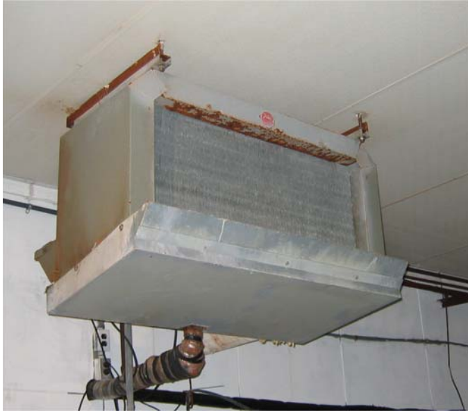
35. Overhead Freezer Air Handler
